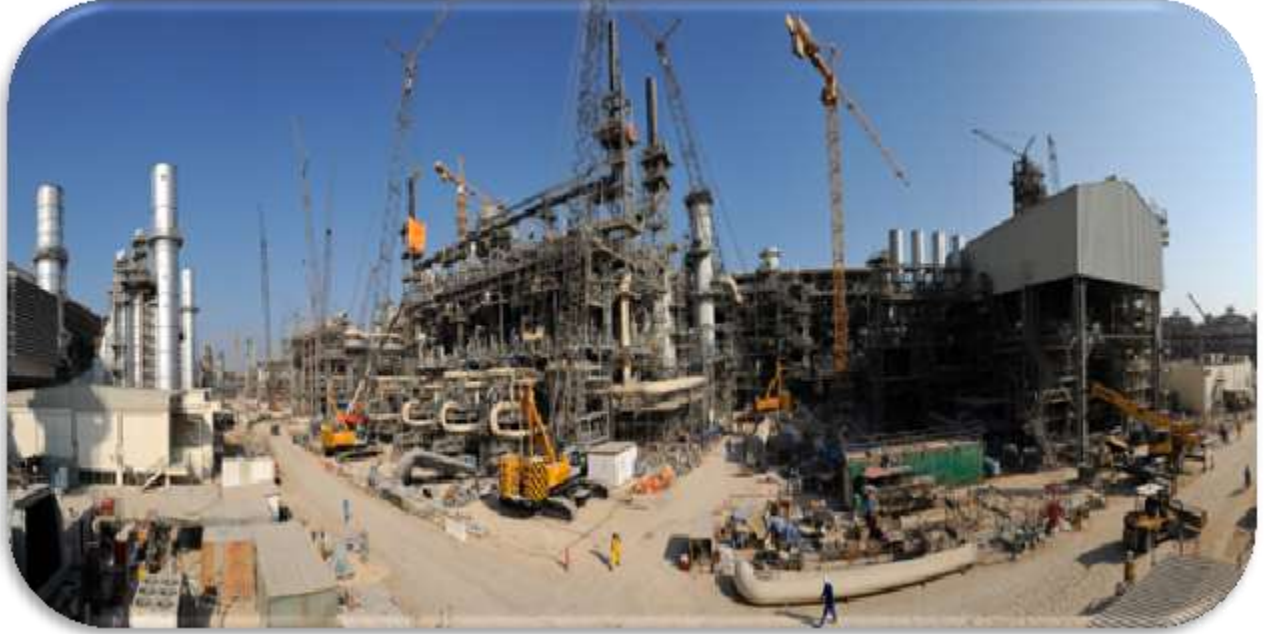
Powering Qatargas. Photo courtesy of Shell.
