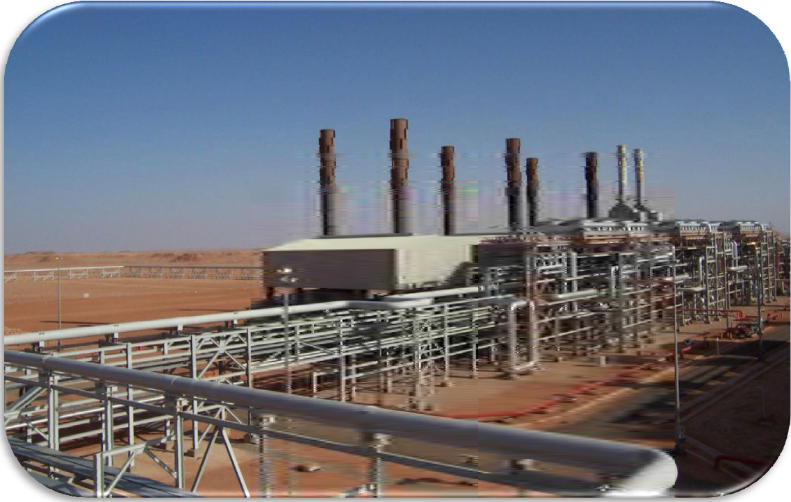
In Amenas gas plant, Algeria. Photo courtesy of BP. See comment on p2
