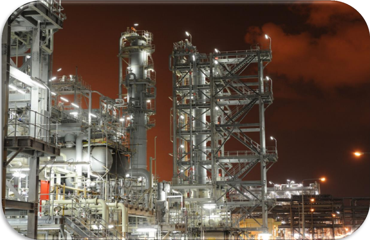
Pearl GTL at night-Qatar. Photo courtesy of Shell.
